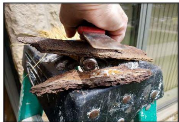
Photo 6 – Close Up View of Removed Rust Pack Measuring ¼" Thick (1/16" Loss of Steel Section)
